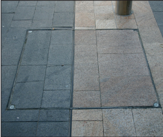
Paving over service covers.
