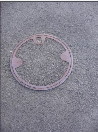
Asphalt over service covers
