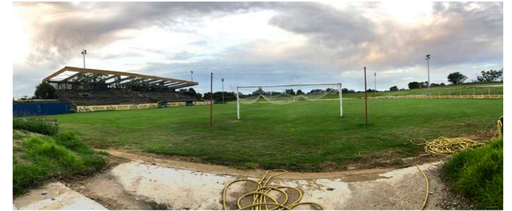
1: Football field and St George football stadium with the damaged roof structure
