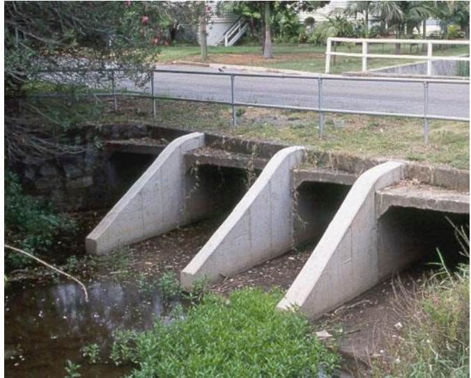
Photo 16: Example of a debris deflector Image Source: Australian Rainfall and Runoff 2019
