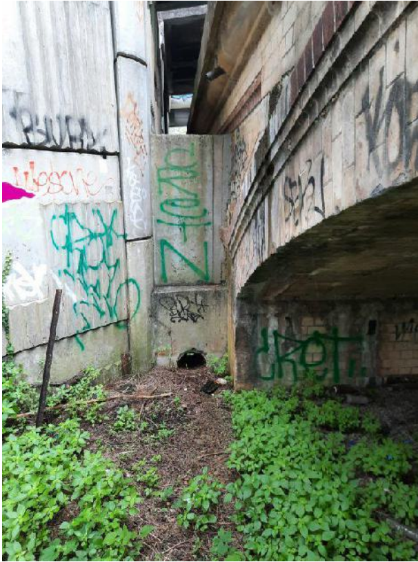
Photo 17: Western opening under the East Hills railway line adjacent to the SWSOOS
