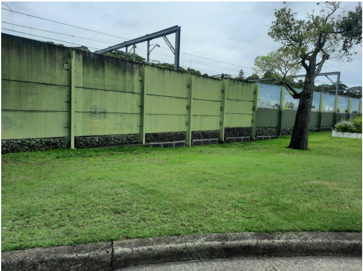
Photo 14: Openings for overland flow under the noise wall at Powys Avenue ( Image Source: WMAwater )
