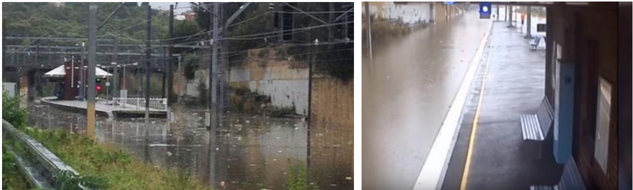
Photo 20: Flooding of Bardwell Park Station in 2015 (Source: Bardwell Creek 2D Flood Study Review , WMAwater 2019)
