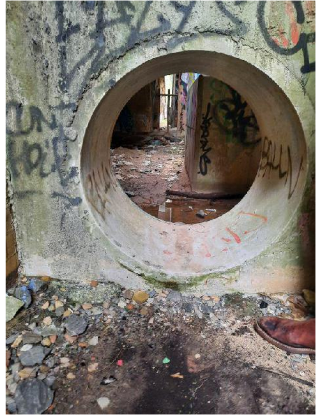
Photo 18: Eastern opening under the East Hills railway line adjacent to the SWSOOS
