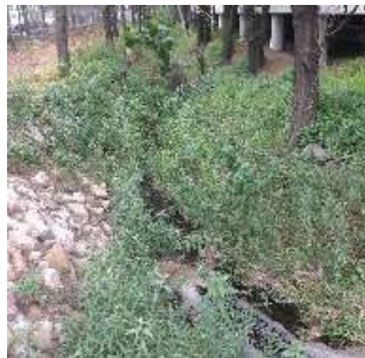
Photo 7 Overgrown vegetation along Floodvale Drain open channel
