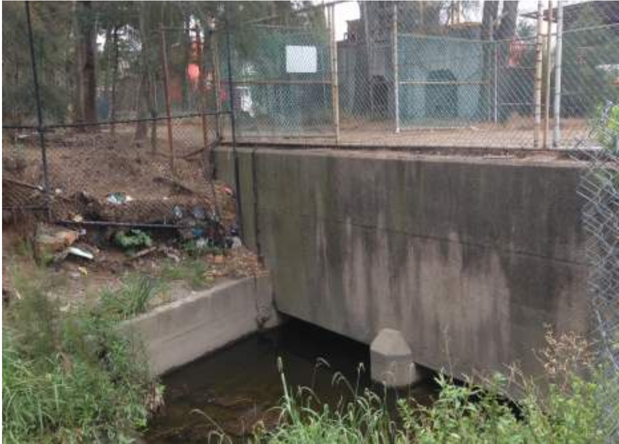
Photo 8 Inverted syphon at intersection of SWSOOS No. 2 and Floodvale Drain
