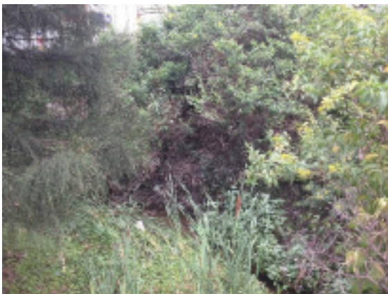
Photo 6 Overgrown vegetation along Springvale Drain open channel
