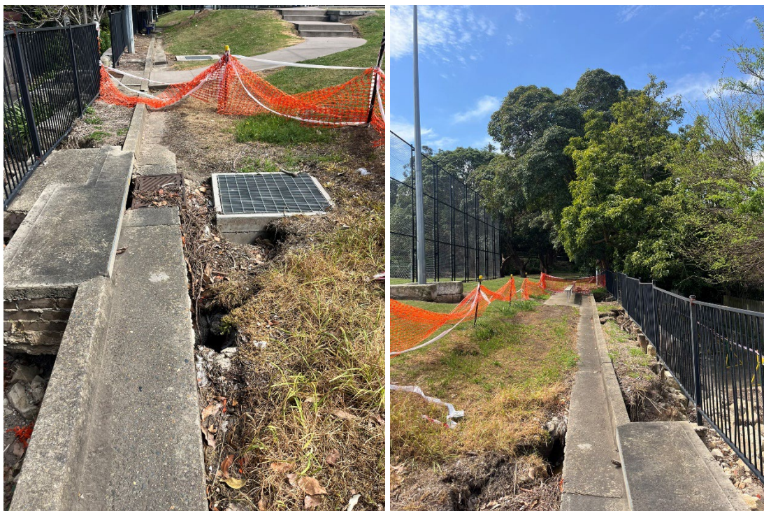
Figure 4-6: Concrete kerb overland drainage system and recently installed drainage pit on the top side of the collapsed segment of retaining wall photographed by RHDHV in September 2024.
