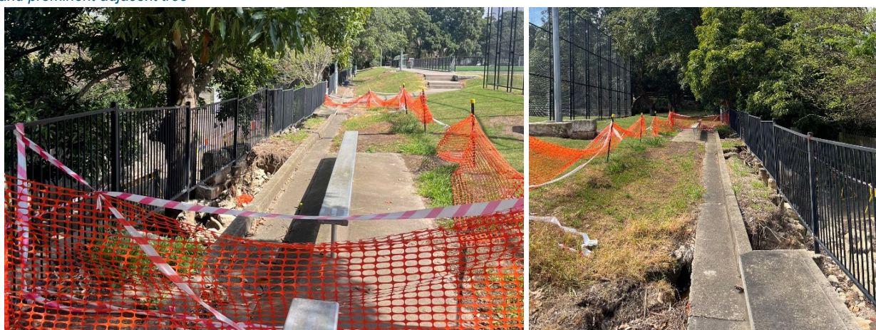
Figure 1-3: Site photographs: Left – Topside of the segment of collapsed retaining wall facing southwest; Right – Topside of the segment of collapsed retaining wall facing northeast
