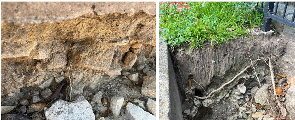
Figure 4-2: Exposed fill material on the top side of the collapsed retaining wall
