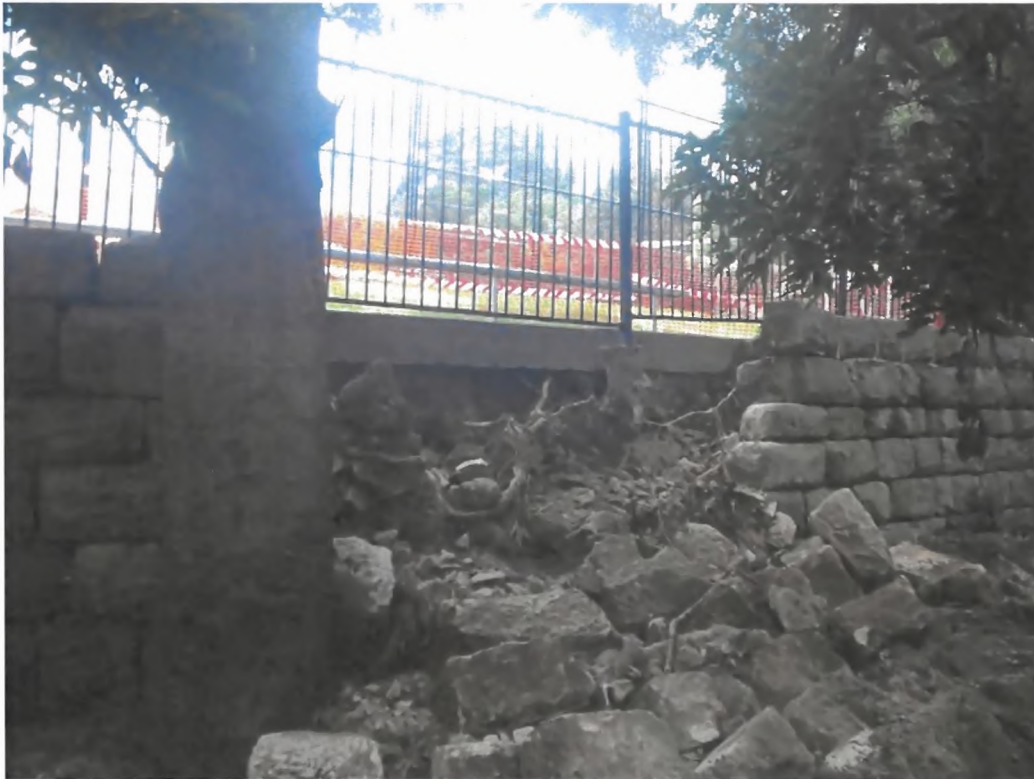
Figure 12 | Looking N at the blocks that have collapsed between the trees. Arborist to consult on the tree roots and tree protection.
