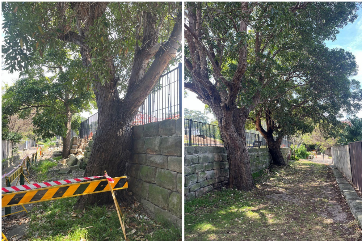
Figure 4-9: Left Photograph – Brushbox and Illawarra Flame Tree located within the proposed retaining wall remediation area; Right Photograph – Brushbox and Green/ Red Ash trees located within part of the proposed site compound area (RHDHV, 2024)
