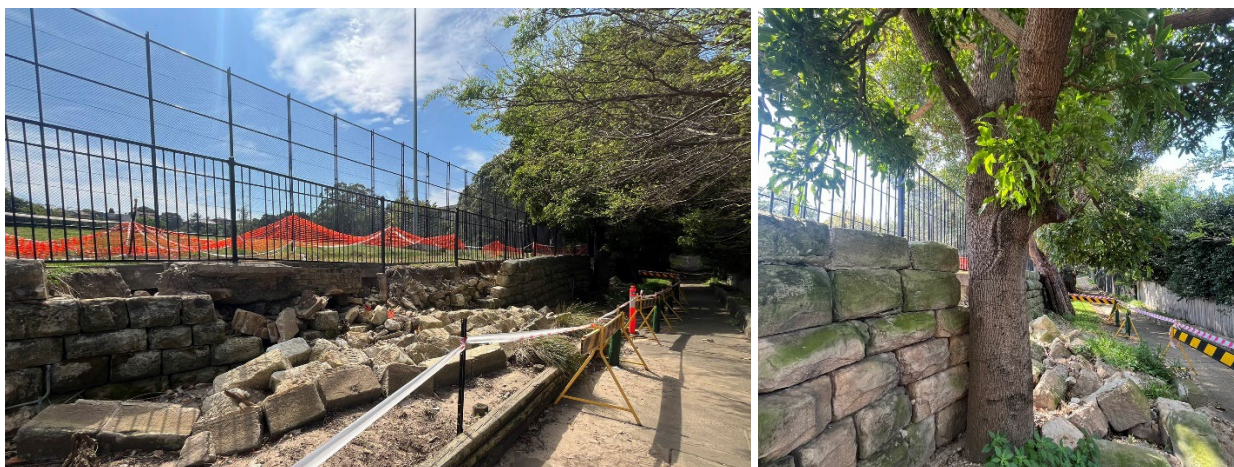
Figure 1-2: Site photographs: Left - Collapsed retaining wall facing northeast; Right – Collapsed middle section of the retaining wall and prominent adjacent tree
