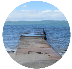
Florence St Stormwater Drain
