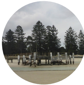
Relic Timber Pier
